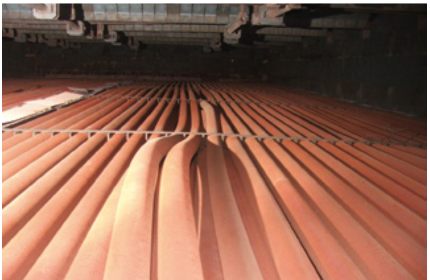
3. Desuperheater overspray contributed to deformation of reheater tubes
