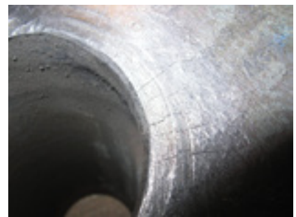
2. Cracking initiated at long weld-neck flange connection also was attributed to excess water
