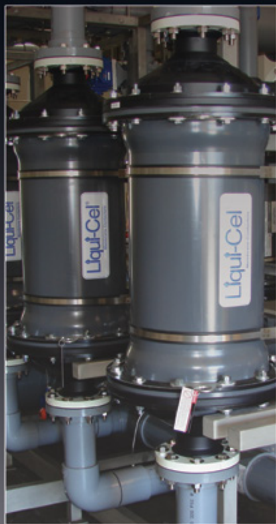
14-inch Degassing System for Corrosion Control
