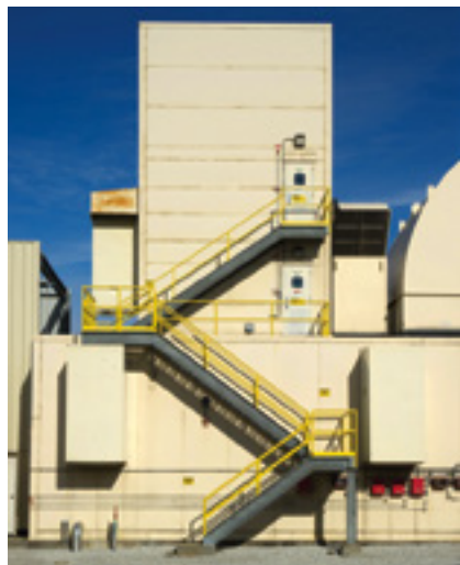
Steps and landings replaced the standard ladder system to facilitate safe access to gas turbine's combustor section. Rokeby Generating Station
