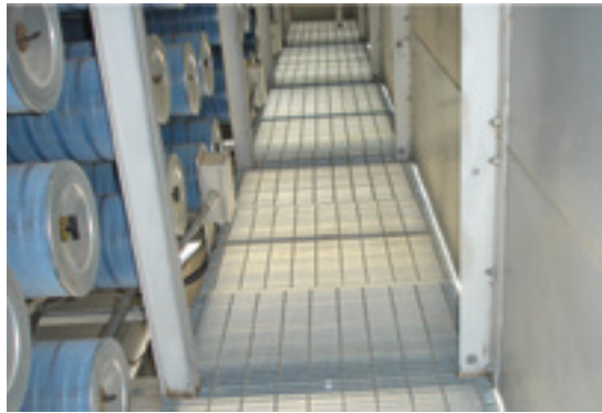
Inlet filter house floor , originally made of steel plate, was replaced with steel deck grating to prevent snow drifting in winter which blocked air flow and to eliminate a slip hazard. Beatrice Power Station
