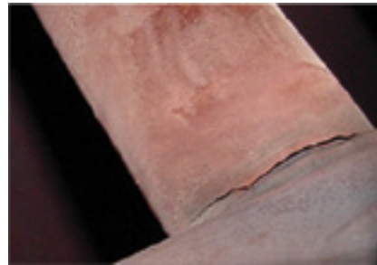
4. Repeated quench of hot tube caused by leaking attemperator control valve resulted in cracking from thermal-mechanical fatigue
