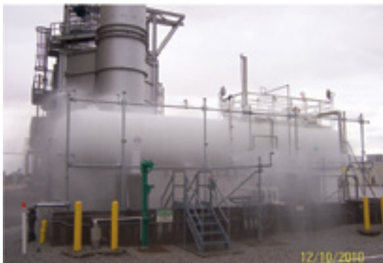
Ammonia-tank leak-suppression system protects plant personnel and neighbors. Water spray system, which has 34 nozzles configured on six lines surrounding the tank, was designed to NFPA
