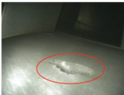
15. Damage to the compressor case was surprising
