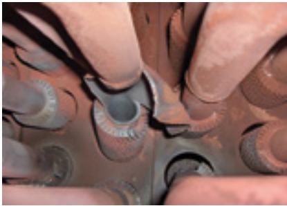
9. Freeze-up of undrained water fractured tubes
