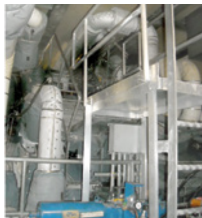
Permanent platform provides safe access to gas-turbine igniters. Granite Ridge Energy
