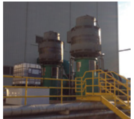
3. No failures are acceptable for two 60% circulating water pumps. All the predictive technology and techniques available are applied to them
