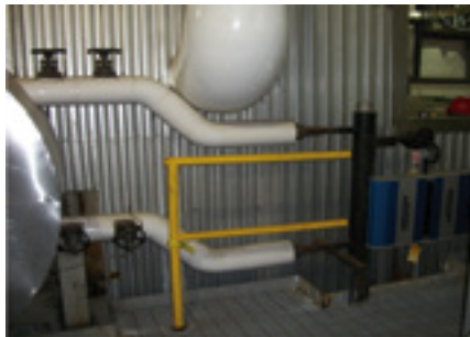
4. Incorrect: Steam and water piping to water column slope downward
