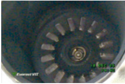
4. Positive impact of atomizing air blower is in evidence after a four-hour run on distillate and oil shutdown
