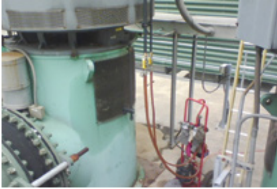
Mobile filter cart and piping modifications allow ground level access to circ-water-pump motor lube sump making hazard-free a job that had been dangerous. Allegheny Energy Units 3, 4, 5
