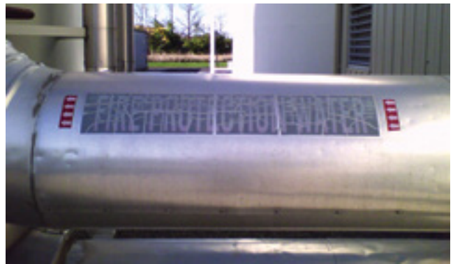
4. ASME A13.1 is the national standard for pipe labeling (left)
