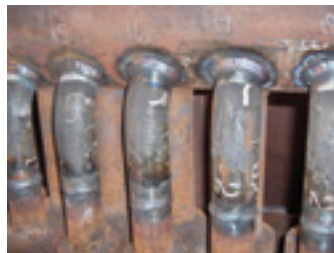
16-17. Improper repair is to cut window out of tube (left); right way is to install dutchman
