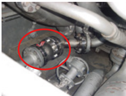
5. Large check valve was installed immediately ahead of the water-injection manifold to prevent air leaking by water-injection check valves from filling the water lines with air when burning gas
