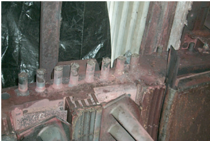
11. Old casings often are damaged during disassembly and reassembly—as these bolts attest
