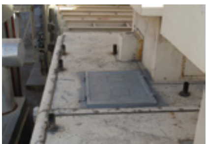
Roof hatch over bearing tunnel facilitates confined-space rescue. Edward W Clark Generating Station
