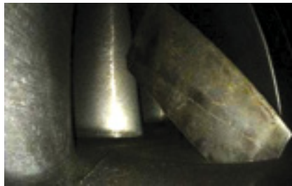
3. Protruding S0 shim located between vane segments five and six
