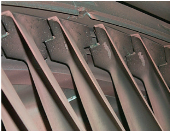
10. Large gaps between third-stage bucket tip shrouds are indicative of loose dovetails
