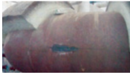
3. Elbow cracked in cycling unit after repeated contact with spray water
