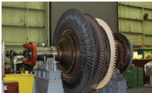
B. Marriage coupling broken , turbine section is prepared for cleaning and the repair of one bucket
