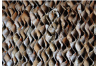
2. Evap cooling media was heavily fouled with contaminants
