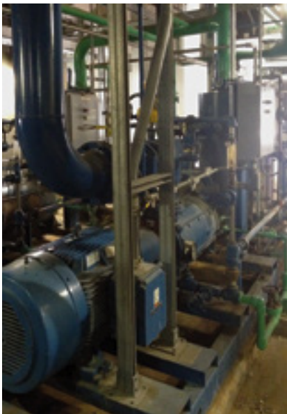
4. Vacuum-pump cooling system was identified through the RCM program as deficient. Modifying it gained 5 MW of output
