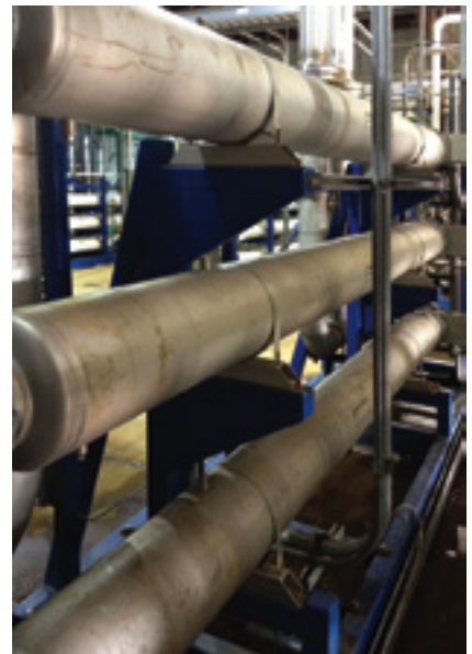
6. High-temperature shutoff system was found missing from the RO pumps. Once the requisite sensors and switches were added, a history of failures was arrested
