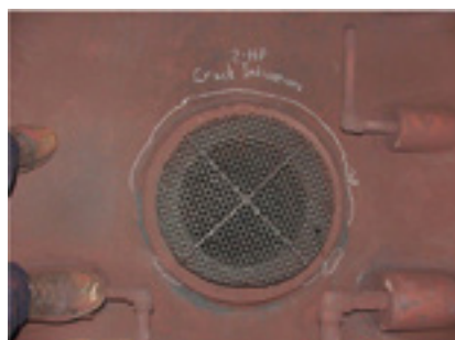
6. Cracking is visually evident at the downcomer-to-drum connection at left; close-up photo of the crack is at right
