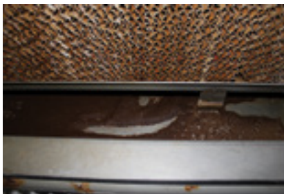
3. Contaminants accumulated in the wetted-media water trough
