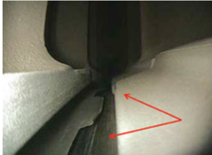
20. Air seal damage shown is significant and relatively easy to miss in a borescope inspection because the material below it resembles an air seal
