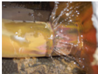
1. Tube leaks can be expected in HRSGs with poor drain systems
