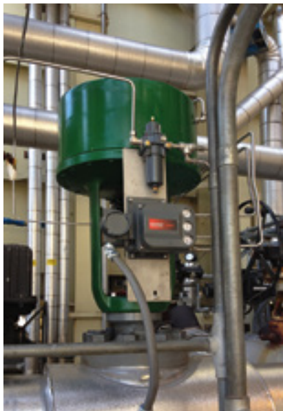
5. Replacing undersized actuators on the HP feedwater and feedwater minimum-flow valves allows the plant to consistently run at heat rates below 7000 Btu/kWh
