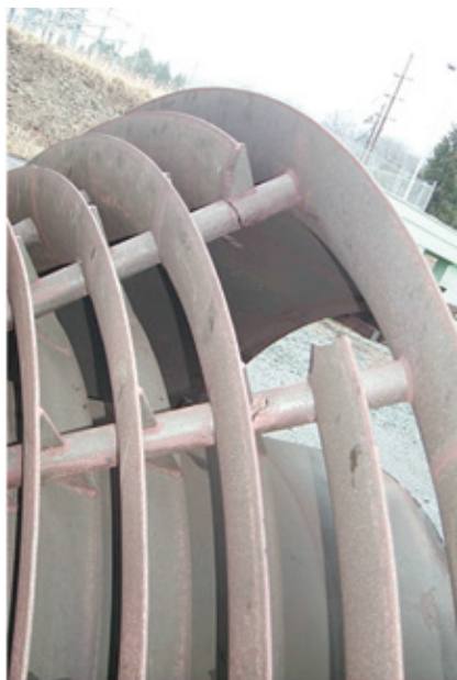
12. Cracking of exhaust-diffuser turning vanes is relatively common in the 7B fleet
