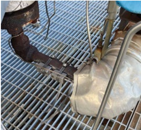
8. Flexim flow measurement between control and block valves
