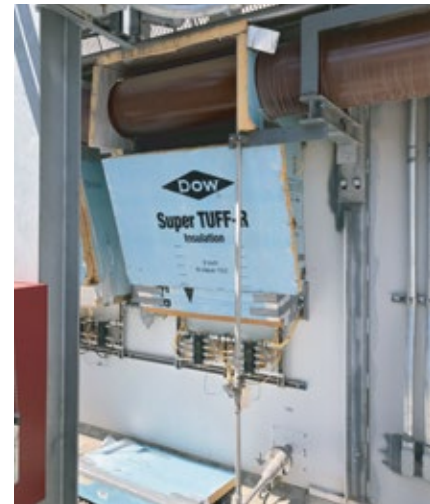
2. Temporary enclosures were fabricated in a manner to capture heat from gas-turbine lube-oil lines
