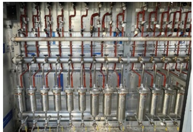
2. New sample panel with primary coolers and double-block-and-bleed valves
