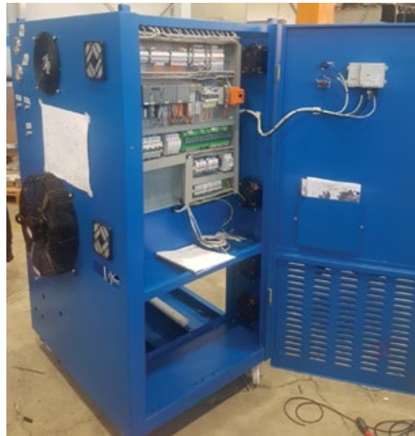
4. A five-year payback for the hydrogen generators at EVM II is expected
