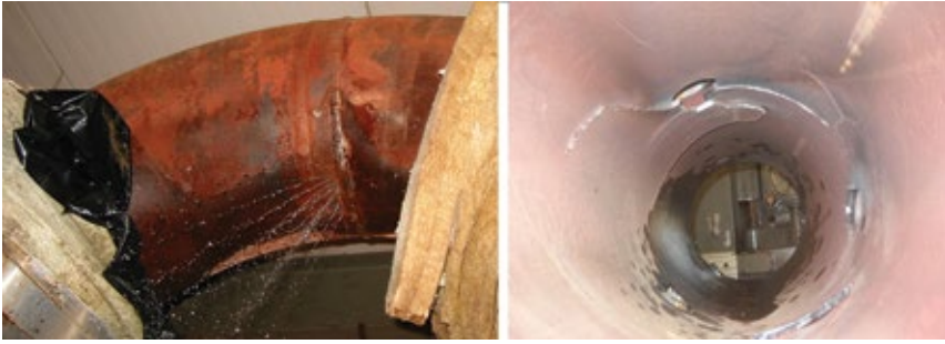
3. Cracked attemperator liners and moisture impingement on downstream bends can occur when attemperation flows are excessive after GT upgrades
