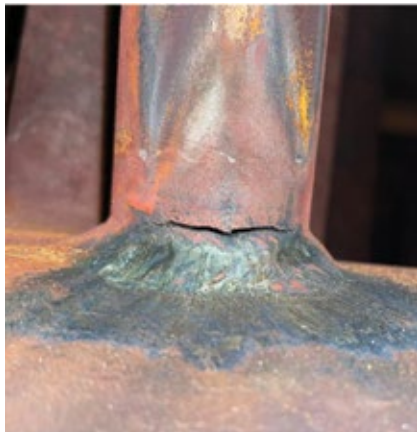
2. Crack associated with the first leak is located on the root of the tube-to-header weld on the tube side. Crack length is about half the tube circumference
