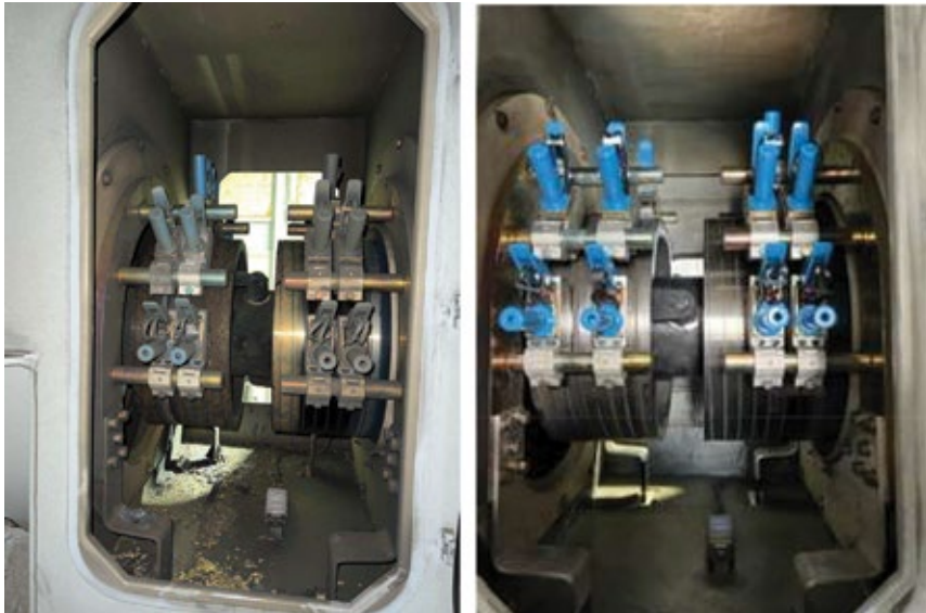
4. Collector-brush flashover (at right in left photo) was caused by inadequate maintenance. Repaired rigging is at right
