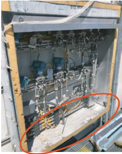
1. Temporary transmitter enclosures with foam-board insulation, made by plant staff, mitigate freezing and other weather effects
