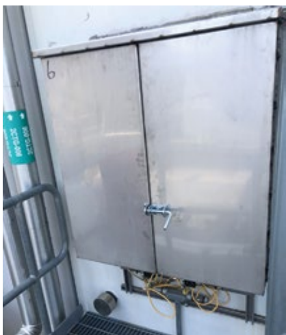
3. Six enclosures were fabricated in-house for each gas turbine. The material: 16-gauge, Type-304 stainless-steel
