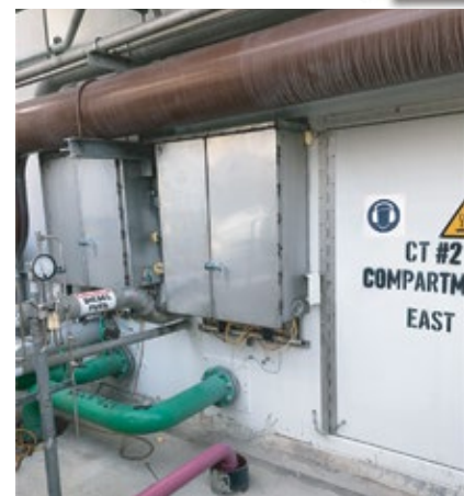
6. New enclosures were field-fitted around existing permanent infrastructure, enabling plant personnel to fabricate and install them with no loss of generation
