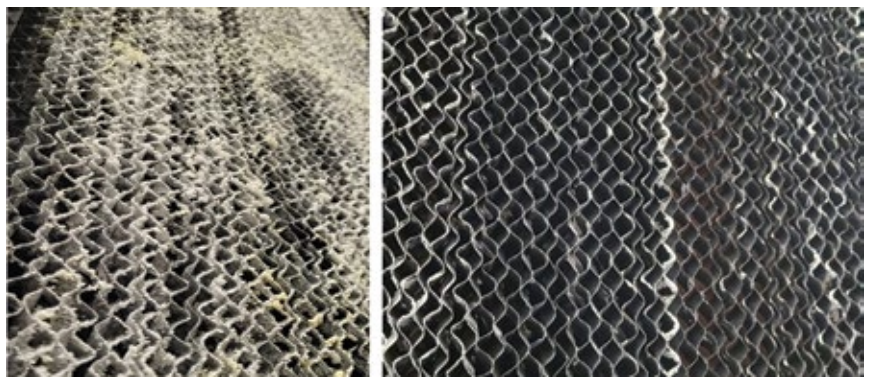
1. Media fouling was significant after operation for one year with poor-quality water (left). Mixing service water with demin achieved the desired result (right)
