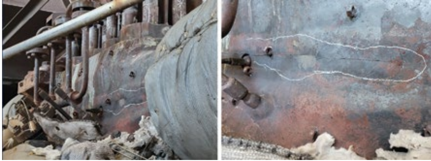
3. Through-wall crack in turbine steam chest, 48 in. long, was one of the more dramatic “indications” causing the presenter to ask, “How much longer can this unit run?”
