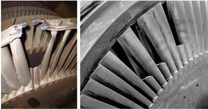
13. Steam-turbine L-0 blade resonance causes high-cycle fatigue damage, leading to blade failure
