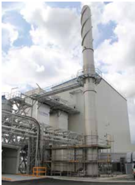
3. 30-MW wood-fired facility in New Zealand
