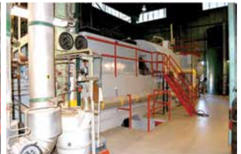
6. Generator is at the left , steam turbine and condenser at the right, looking down the combined cycle on the operating floor
