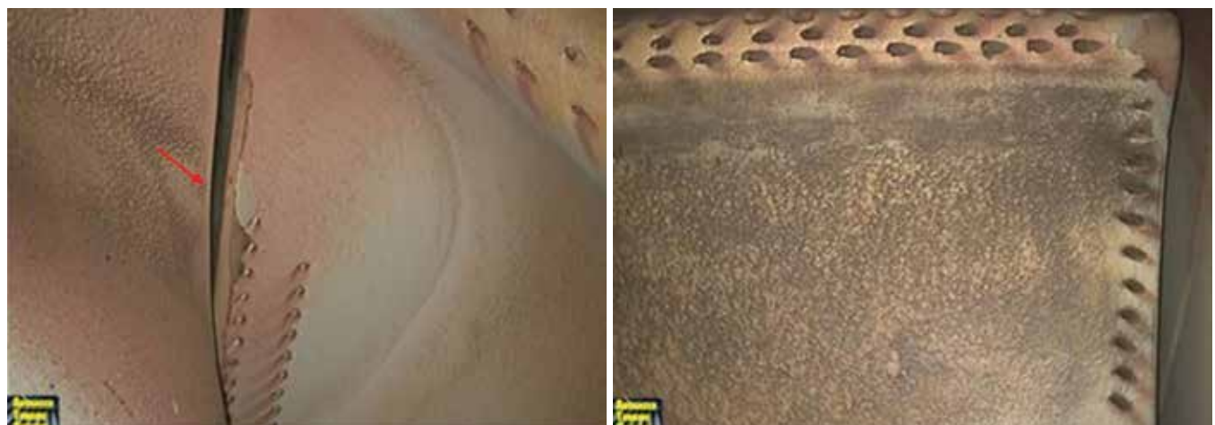
8. Coating loss at the platform edge is seen in the left-hand borescope photo; leading-edge tip coating loss and discoloration at the right
