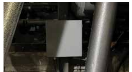
4. Junction box was relocated to keep t/c wiring out of harm's way
