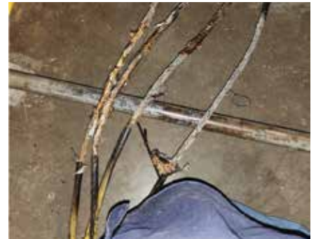
3. Leak in the transition-piece steam supply system damaged thermocouple wiring
