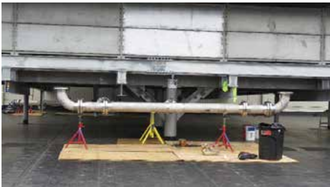
2. Anti-icing header is located below the filter house
