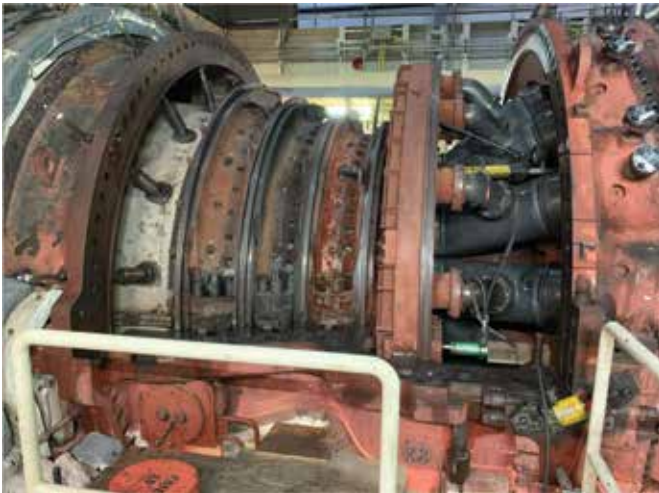
Excessive base-metal oxidation in Rows 2 and 3 encouraged the unit owner to plan for blade-ring exchanges
