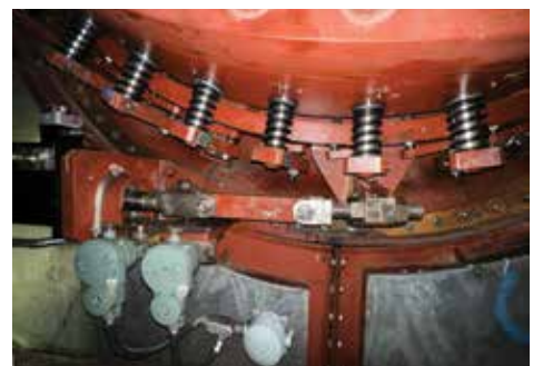
Remember to verify linkage thrust force after lubricating your IGVs
