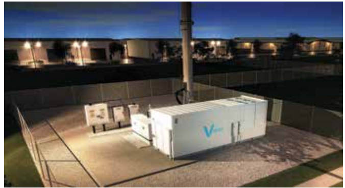
ORR Protection Systems provided 501F and 501G users a useful primer on lithium-ion battery technology
