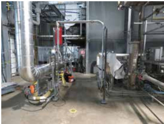
6. Control valve and instrumentation underpin the anti-icing system
