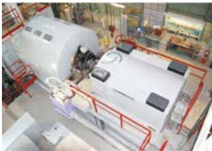
4. Looking down at the combined cycle the gas turbine is at the left, generator at the right
