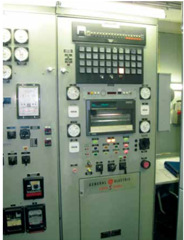
Speedtronic™ Mark I control systems were installed on gas turbines in the early 1970s, primarily on MS5001N and MS7001B engines
