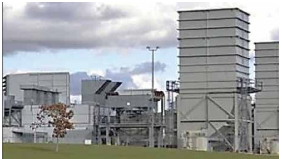
SVI/Bremco’s presentation demonstrates reliable ways to upgrade simple-cycle-turbine intake and exhaust systems using one-dimensional algorithms, CFD, and other methods
