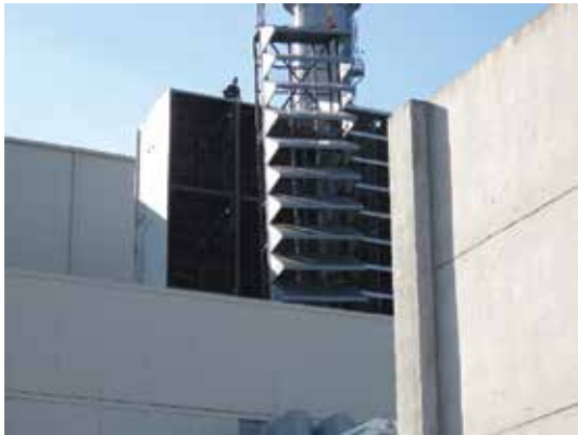
5. Anti-icing module is lowered by crane for installation in the filter house
