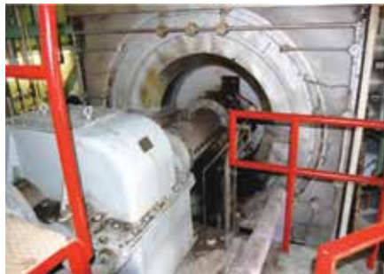
5. Gas-turbine exhaust end is to the right of the reduction gear
