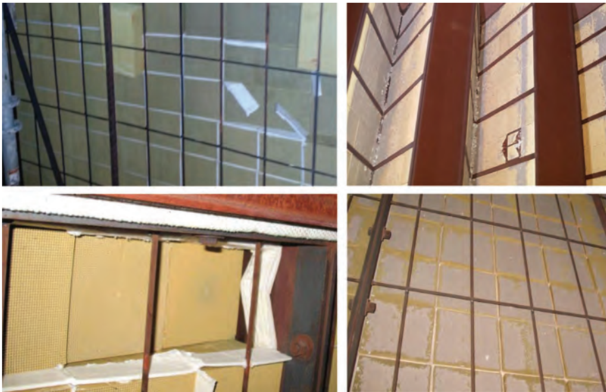
5. Visual inspection of SCR catalyst shows critical need for maintenance (cleaning, repacking, restacking) to restore lost performance from plugging and structural issues
