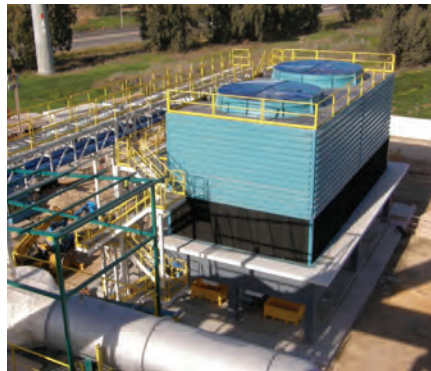
1. Cooling tower serving the gas-turbine inlet-air chillers is critical for producing maximum power
