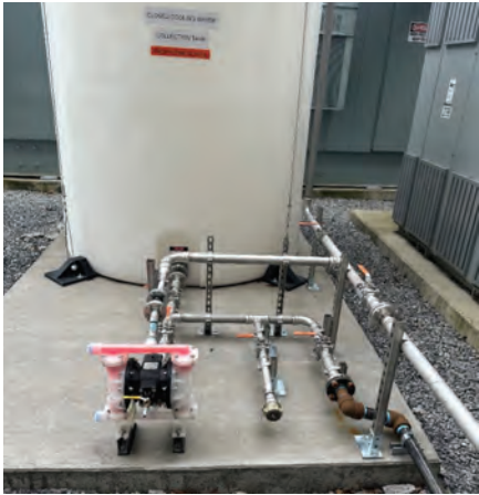
2. Holding tank is supported by a fluid system consisting of permanently mounted valves and pump
