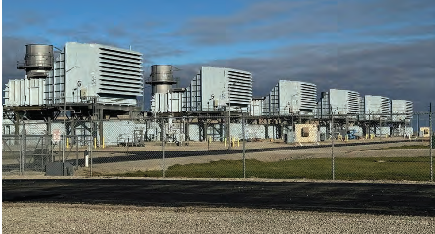
1. Generating plant features multiple 7EA simple-cycle peakers
