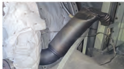
1. Location of IBH flex hose failures is indicated by arrow in the drawing; a flex hose failure is shown in the photo
