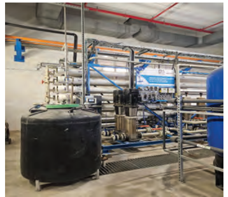
4. Water treatment system can produce 60 gpm RO water and 70 gpm of demin water
