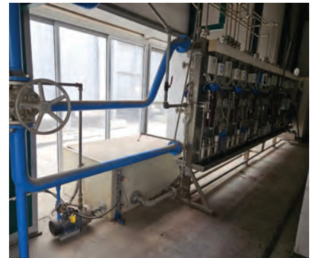
3. Water collected from the steam-quality monitoring system is sent to the cooling tower
