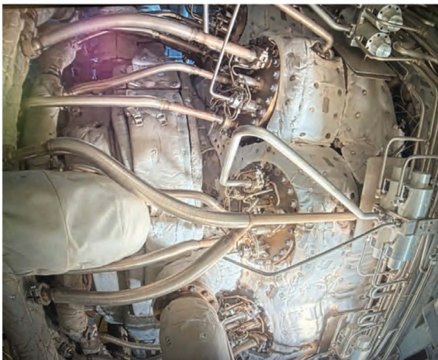
2. Visual of combustors as seen by control room operators
