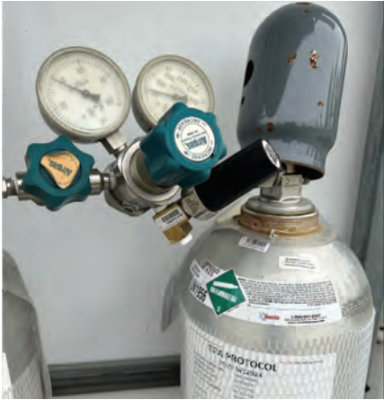
1. Calibration-gas consumption is measured in real time by sensors mounted on the tank as shown
