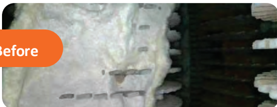
Before cleaning 8th row of tubes
