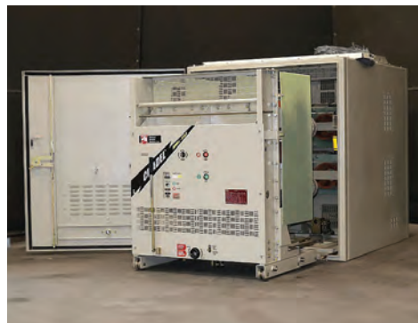
3. Circuit breaker at right is inserted into the cell at left
