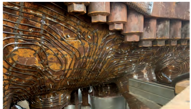
8. Permanent placement of redundant sets of heating wires on the casing below the split line, plus the use of a heat-reflecting shield over the wires, assures optimal effectiveness and reliability of the warming system
